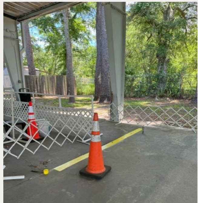
The shifted concrete in Ring B has been painted yellow.
